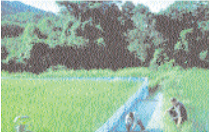
Grant Singleton advising on the construction of a community trap barrier system in Luang Prabang, Lao PDR. The mound of mud leads to multiple capture traps.
